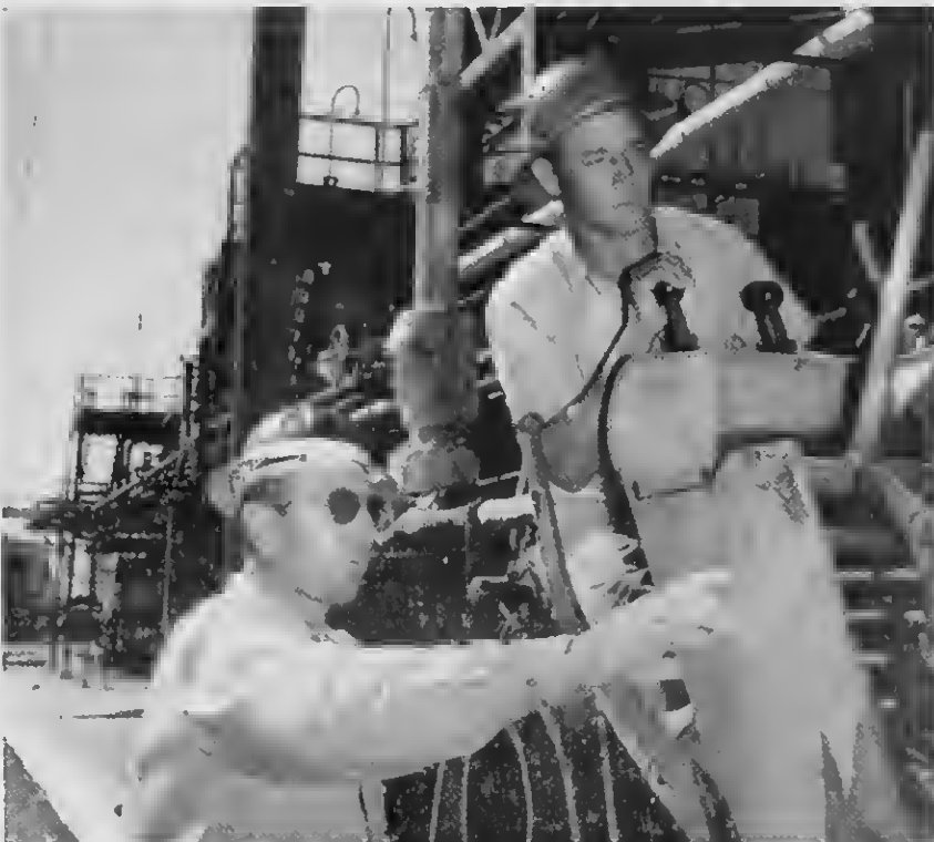
RIGGER-FOREMAN Moritz gives instructions to crane-operator Wernet. RIGGER-FOREMAN Moritz ta duna instrucion na operador di grua Wernet.
